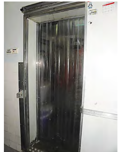
Install strip curtains
